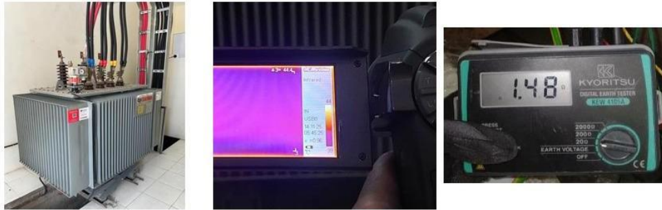
Gambar 2. Kondisi fisik transformator, hasil thermography (44,4°C), dan hasil pengukuran grounding transformator (1,48 Ω)
