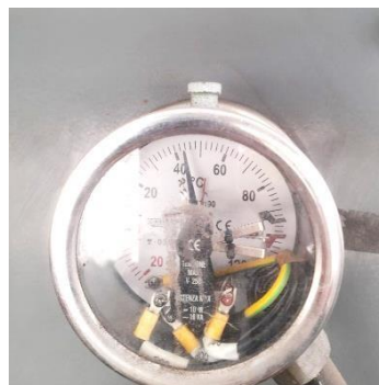
Gambar 10. Foto Oil Temperature dan Winding Temperature
