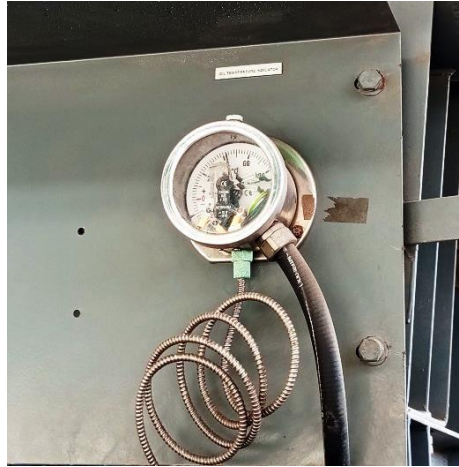
Gambar 3. Foto Oil Temperatur Indicator Transformator TR 5-2
