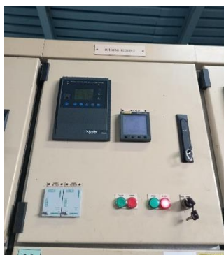
Gambar 7. Foto Monitoring Over Load Relay
