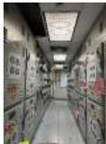
Gambar 3. Motor Control Center (MCC)
