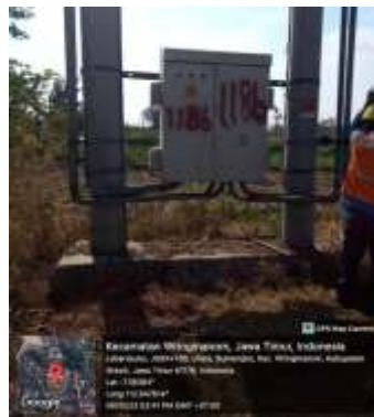
Gambar 1. Gardu Distribusi PHB-TR
